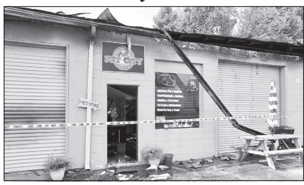
Pet City USA on Old Blue Ridge Highway suffered damage after a fire spread in the building's attic. Photo by Shawn Jarrard
